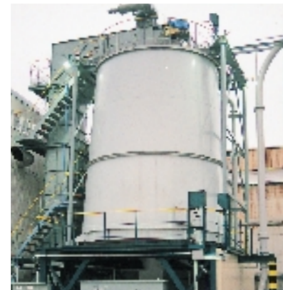
Waste Plastic-to-Fuel Recycling Plant
