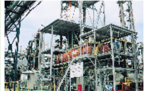
Waste polyvinyl chloride recycling plant
