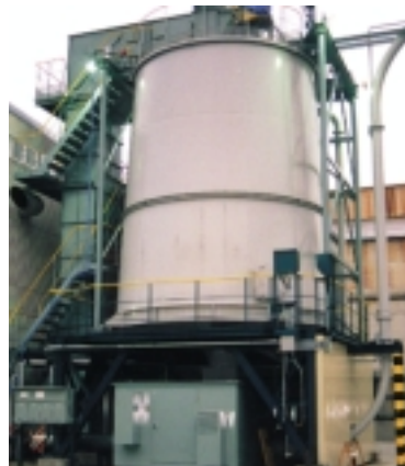
Waste Plastic-to-Fuel Recycling Plant
