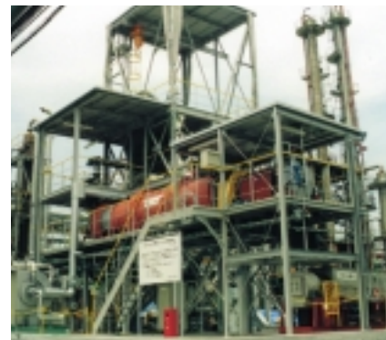
Waste polyvinyl chloride recycling plant
