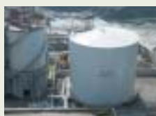
Facility to accept waste film developer
