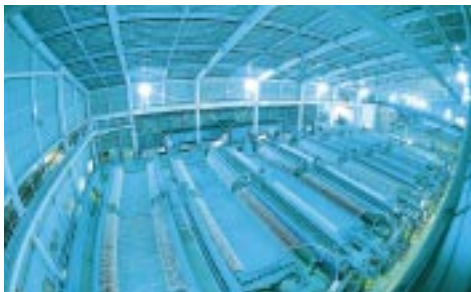
Tokuyama's electrolytic caustic soda plant.
